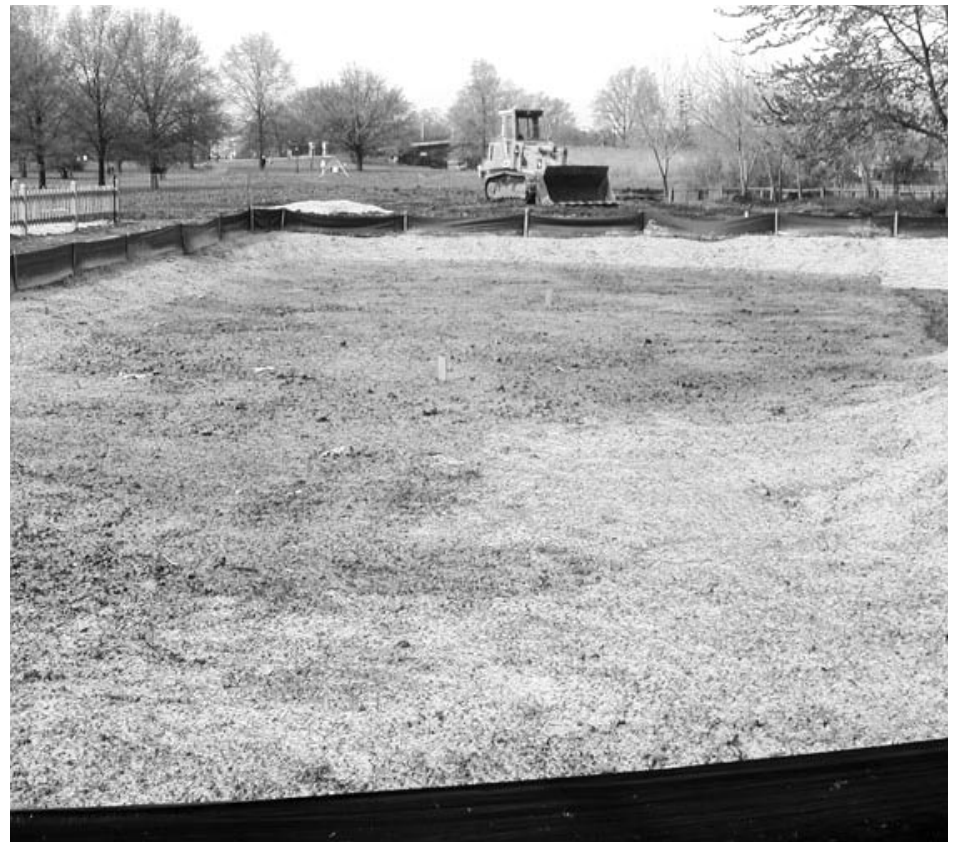
Freshly Seeded Bioswale (landscape with amended soil and selected plants that manages stormwater onsite)
