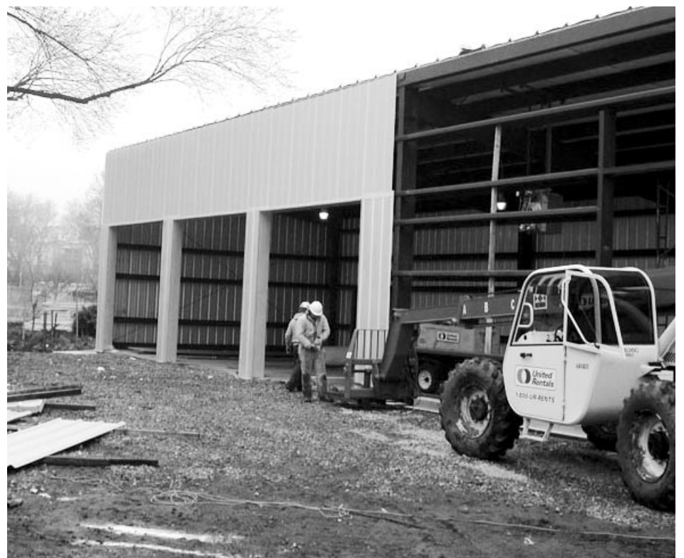
Installing Translucent Panels on New Horticulture/Maintenance Building to Invite Natural Light into Workspace
